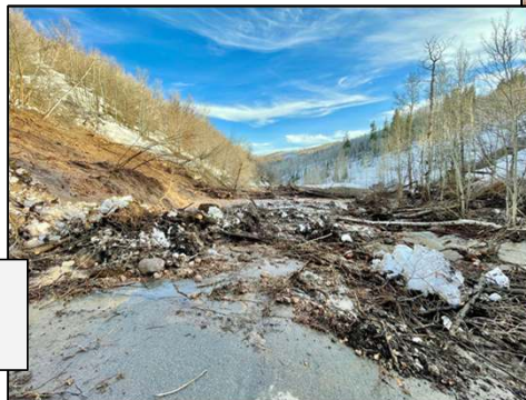
Mudslide area on upper Tollgate Canyon Road
